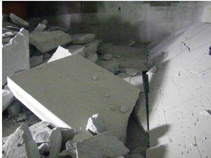
Figure 1. 100 t furnace severely damaged by a steam explosion in 2015 during dry-out [2].
